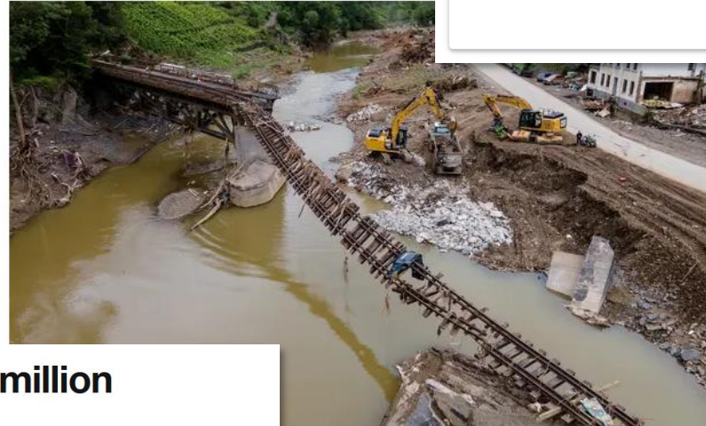
for the flooding of the River Ahr in Rech in the Ahrweiler district of mann Vogel/EPA
